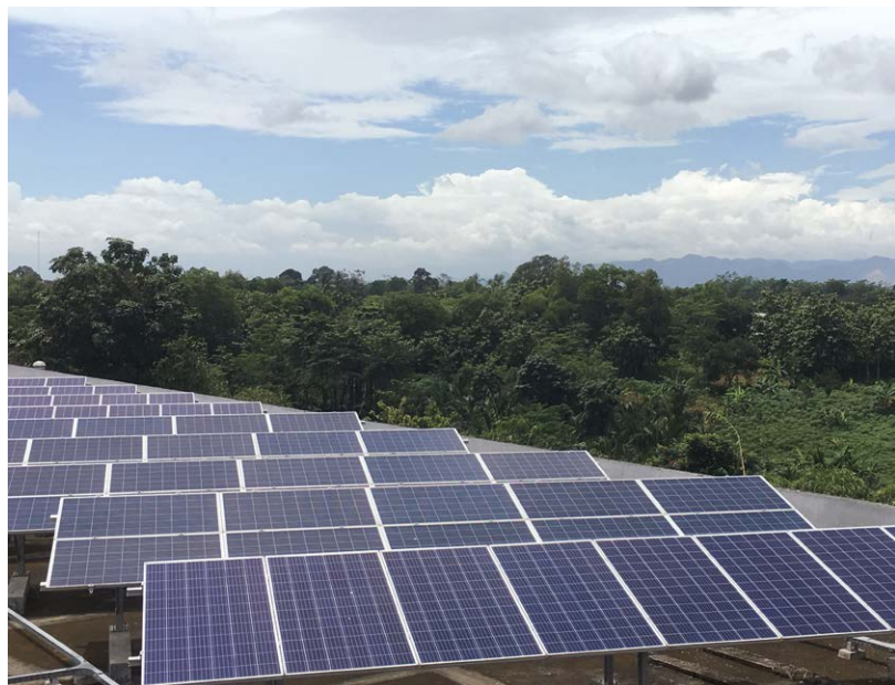
Roof-mounted photovoltaic system in Jakarta, Indonesia
